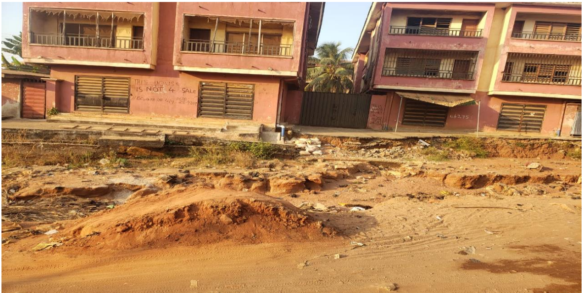
Figure 10. Site of gully erosion on Akwakuma-Umunyali road Owerri-Mbaitoli road, Imo State, Nigeria(Photo taken by the researcher on 13th January,
