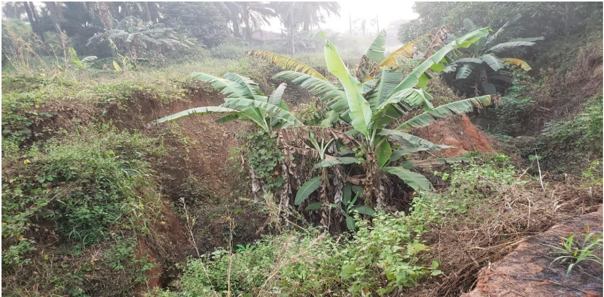
Figure. 9 Gully erosion around Ebom –Umuahie road in Mbaitoli LGA(Photo taken by the reseaecher on 12th January, 2023 at Mbaitoli LGA, Imo State).
